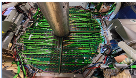
The installed Readout with services in the cavern of ALICE pit
